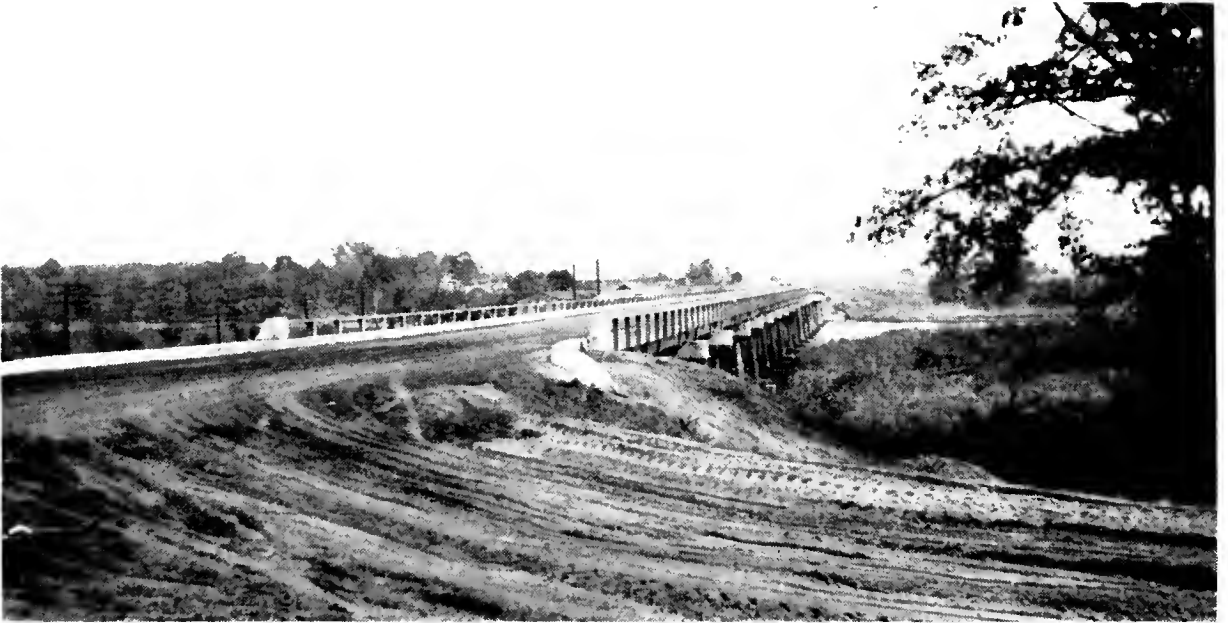
BRIDGE OVER TUCKAHOE CREEK ON ROAD FROM EASTON TO DENTON, CAROLINE-TALBOT COUNTY LINE. UNDER CONSTRUCTION JUNE 30, 1948
